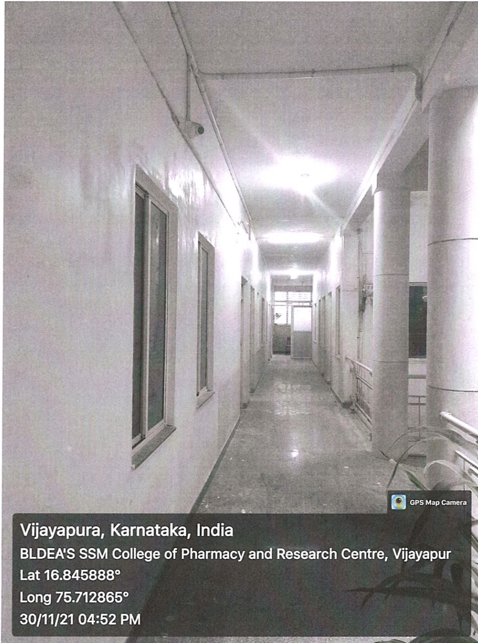
First Floor CCTV camera
