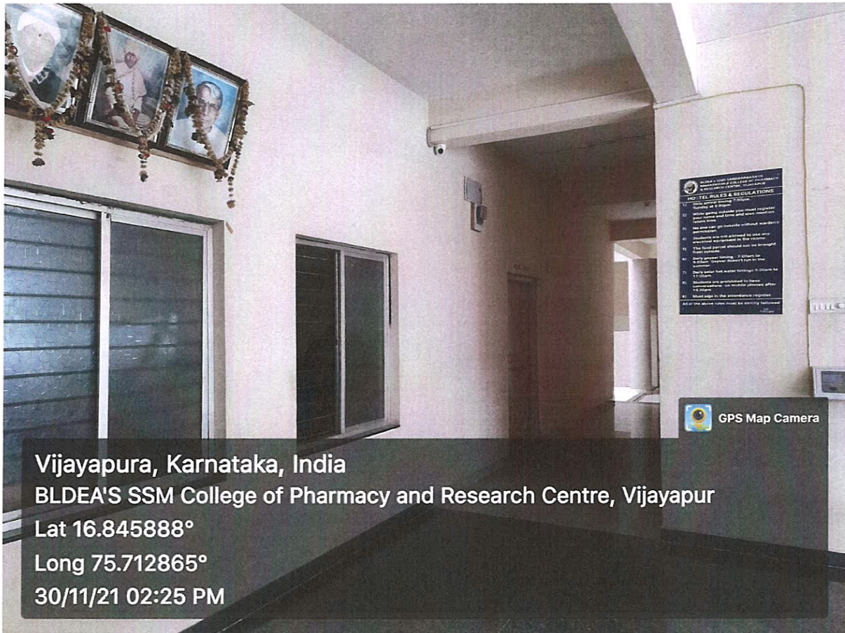
CCTV Camera at Girl's Hotel
