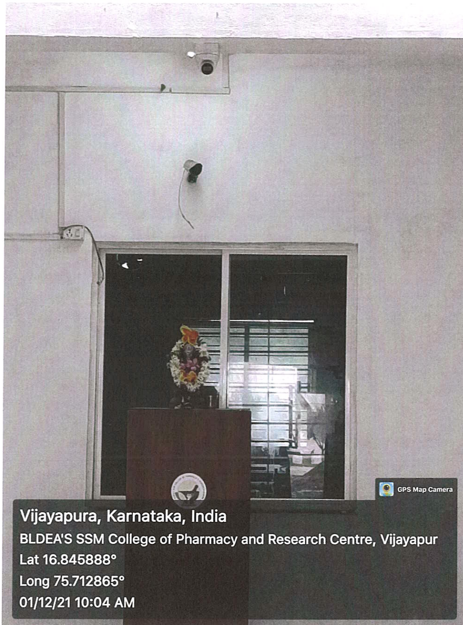
Ground Floor CCTV camera
