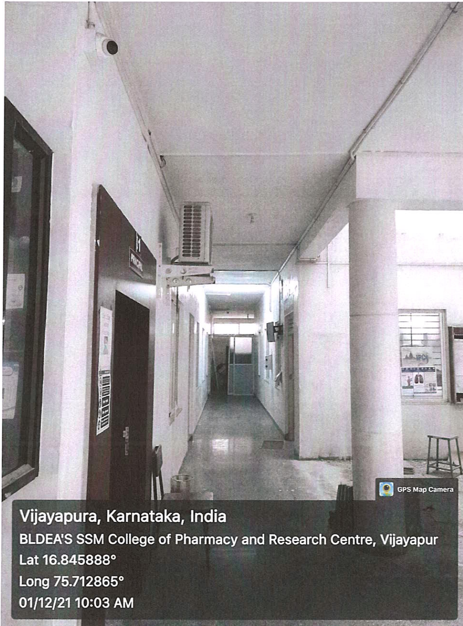
Ground Floor CCTV camera
